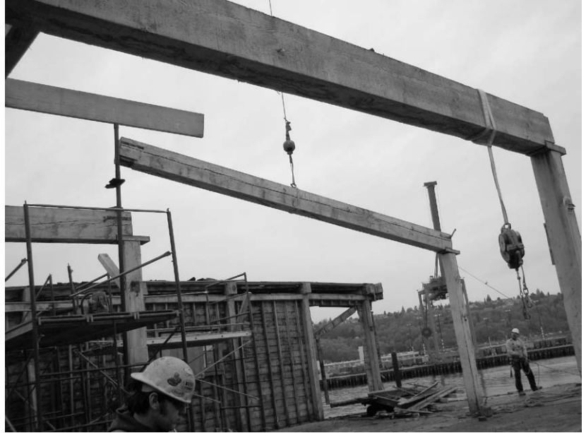
photos these pages Kinley Deller Careful removal of a beam from the second floor of a 1905 warehouse.
