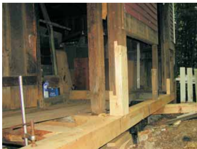
A typical fix for a rotten post bottom. Dan Boyle
