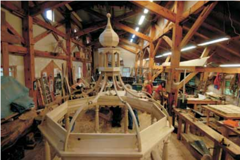
The crown of the bimah replica, under construction in the Handshouse workshop.
