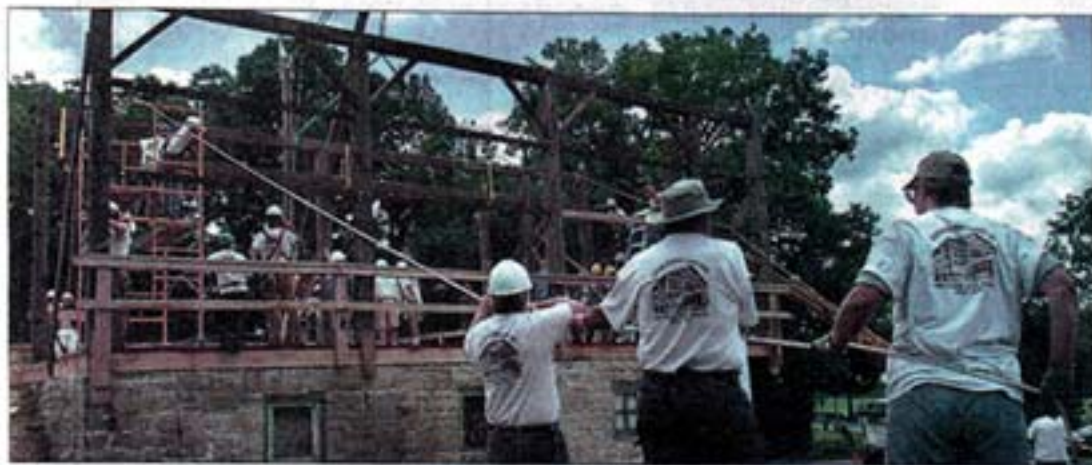
More than 50 people, led by members of the Timber Framers Guild hand-raise a portion of the barn.
